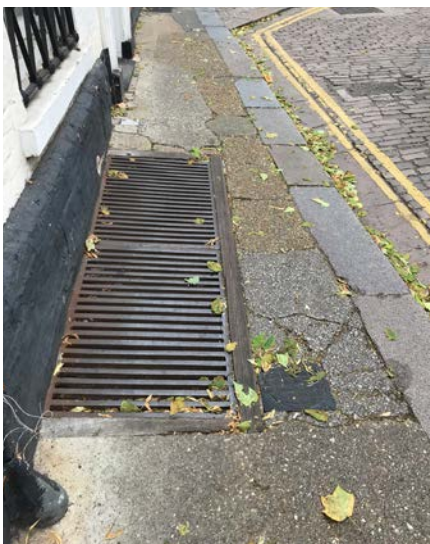
15 - Trip hazard - uneven surface and metal grate - incline 1:8 along Princes Street
